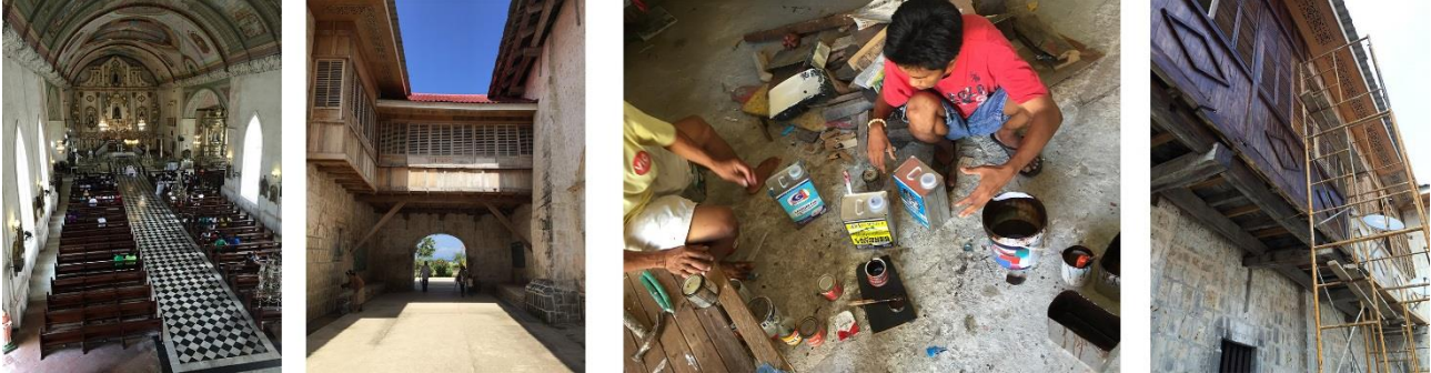
Picture 12. Visit to restoration works in Dalaguete church, south of Cebu island
